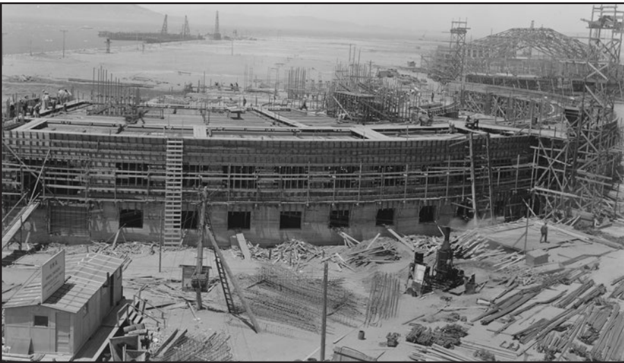
Photo I. This is a view of an air terminal building under construction on the Yerba Buena Shoals Fill — now known as Treasure Island in San Francisco Bay. After completion, the buildings were used as exhibit halls during the 1939 Golden Gate International Exposition. (Courtesy of Wikimedia Commons)
